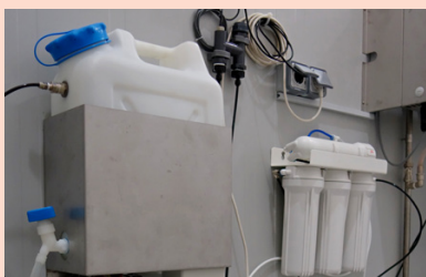
Water Treatment systems
