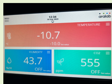
CO2 control and monitoring
