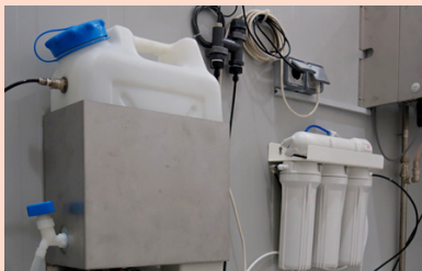
Water Treatment systems
