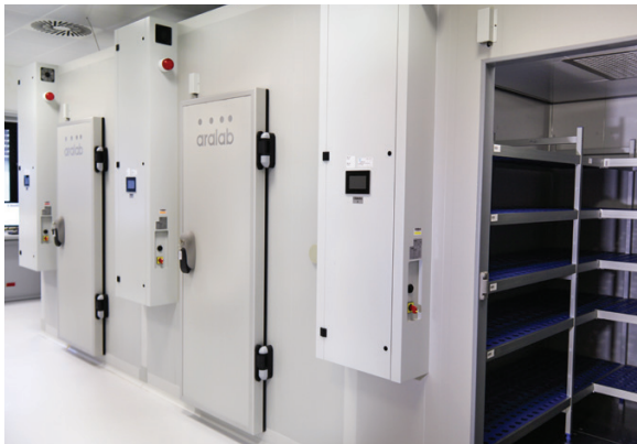
STABILITY ROOMS TURNKEY PROJECT BY ARALAB
