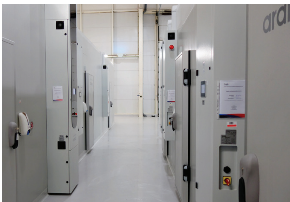
SET OF 8 X STABILCLIMA STABILITY ROOMS AT A STABILITY SERVICES COMPANY
