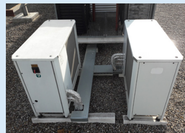
Back-up redundant systems
