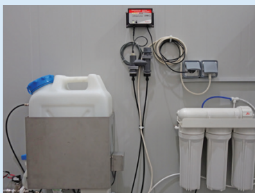
Water treatment systems
