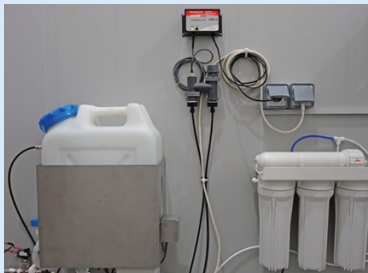
Water treatment systems
